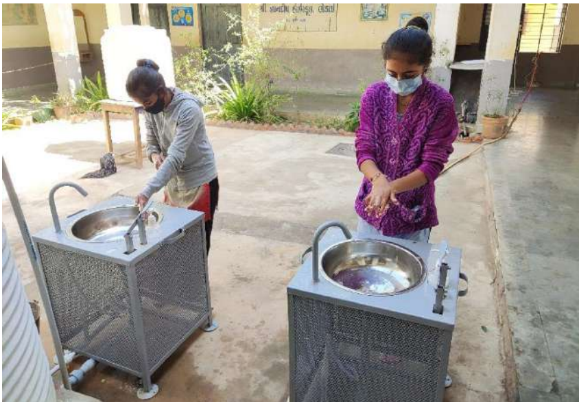
Foot-operated Handwashing Station in use by students at Gyandee High school.
