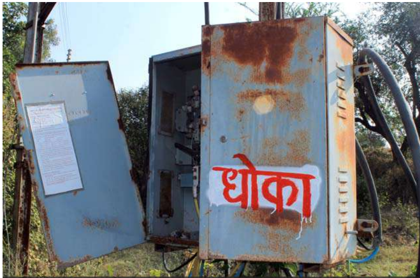
Hazard hotspot: Electric DP.
