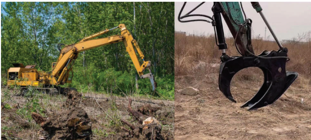
Tree stump removal and land leveling. After poplars are cut, their stumps are removed with specialized diggers. Also refer to Figure 4 for cross-sections of pre- and post-recontouring (photos by ADB).
