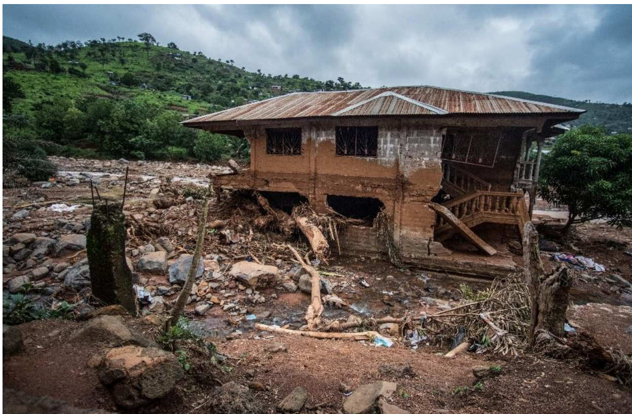
A ruined house a little way down the valley from the mudslide. The brown mark shows how high the torrent of mud and water came up. Photo credit: Olivia Acland
