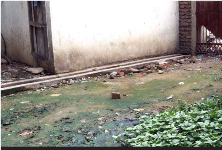
Unhygienic conditions in hospital premises.
